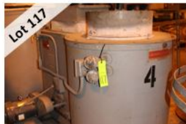
LINDBERG 12-EC-1620-12 ELECTRIC PIT FURNACE
